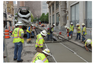
Crews pouring concrete along track placement on Peachtree Street from Auburn Avenue to Ellis Street.
