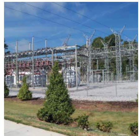
This power substation is classified as TCU-utilities.
