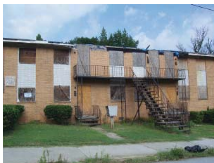
Multi-family residential in deteriorated condition, NPU L.
