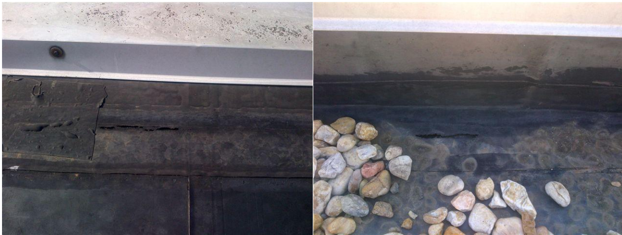
Tears in City Hall Roof Membrane
