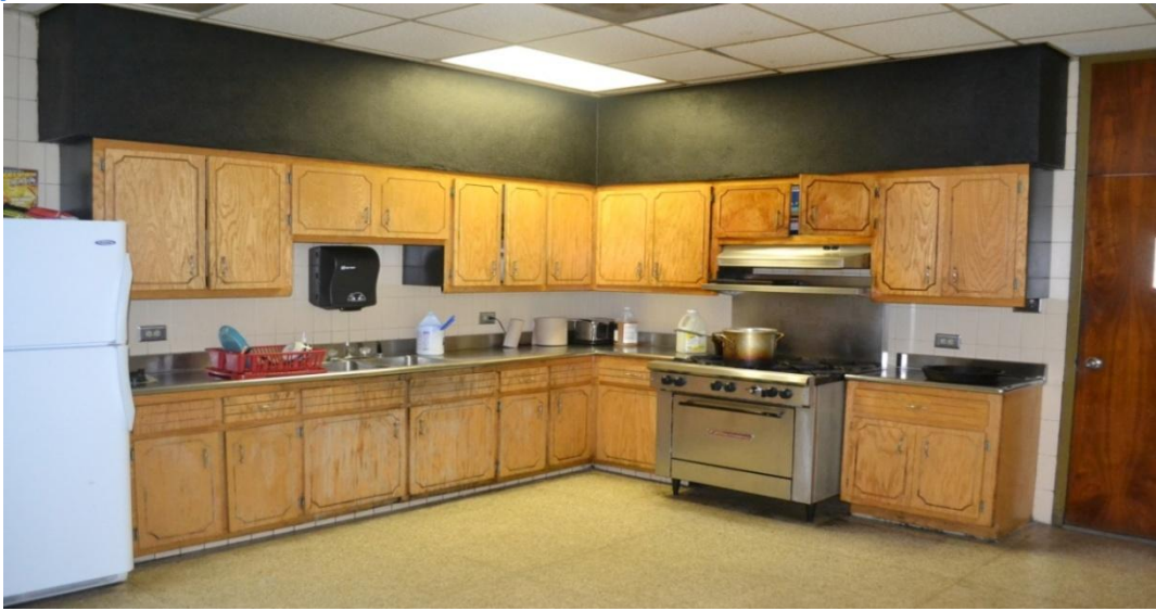
Fire Station Kitchen in Need of Renovation
