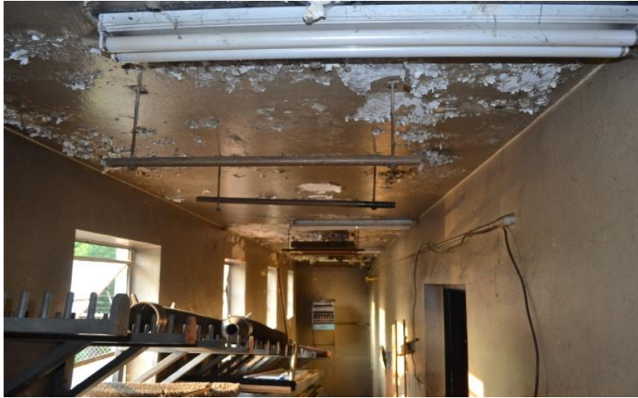
Damage to ceiling at Fire Station 23
