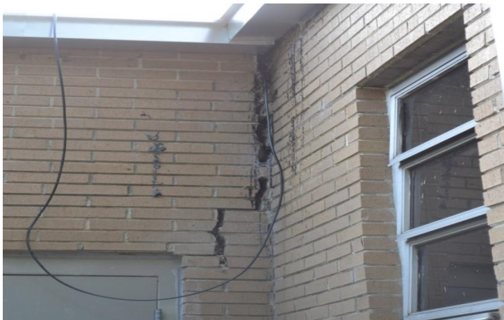
Damage to wall at Fire Station 8
