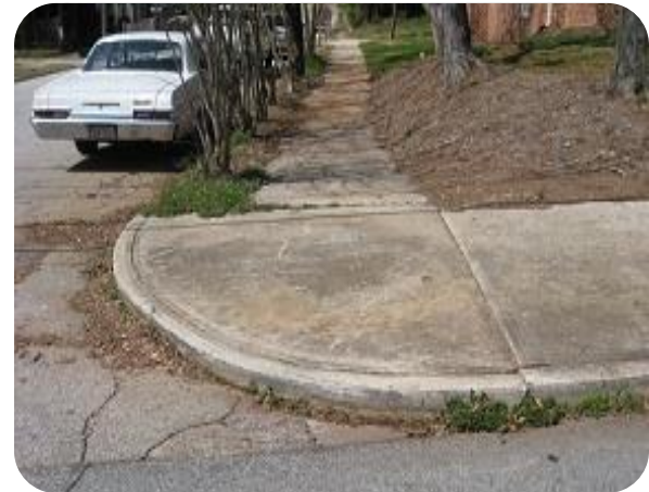
Intersection Node with Missing ADA Ramp
