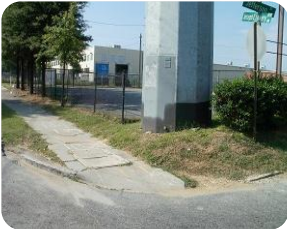
Intersection Node with Non-Compliant ADA Ramp
