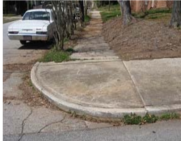
Intersection Node with Missing ADA Ramp
