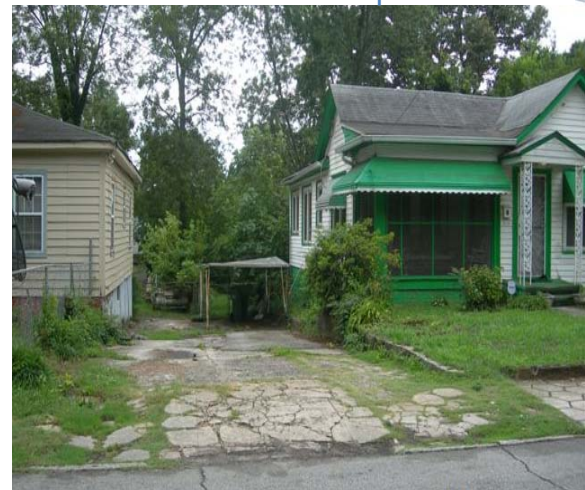
Deteriorated & Non-ADA Compliant Sidewalk
