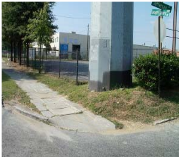
Intersection Node with Non-Compliant ADA Ramp
