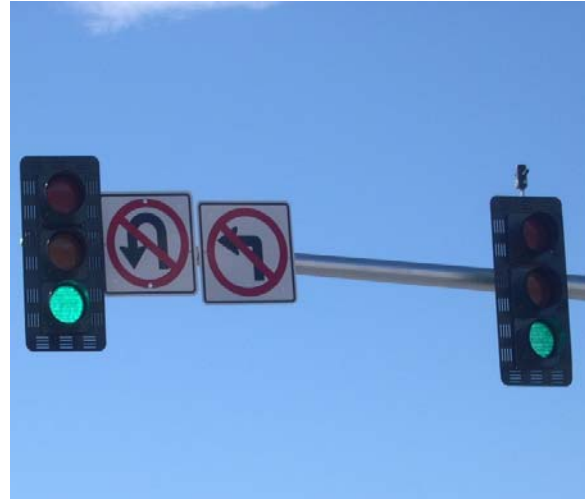
Upgraded Traffic Signal
