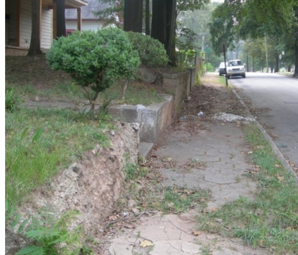
Deteriorated & Non-ADA Compliant Sidewalk
