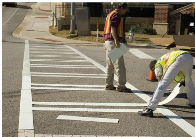
Crosswalks should be repainted where they are worn, substandard, or non-existent.
