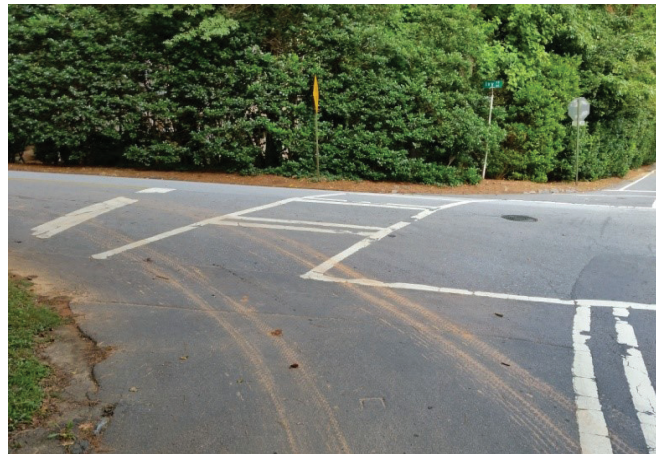
Poorly maintained streets and oddly-placed crosswalks are found throughout the neighborhood.
