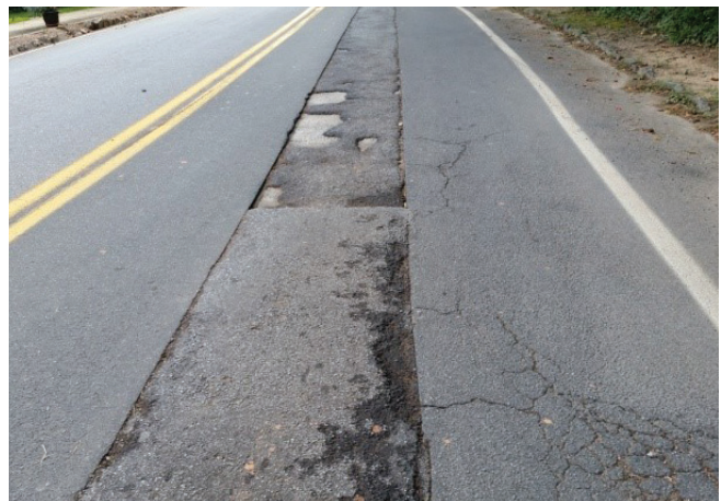
Patchwork done on many neighborhood roads does not comply with the City's Right-of-Way Manual, which requires the entire lane to be resurfaced when cuts are made.
