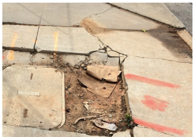
Some sidewalks in the neighborhood are in need of repair.
