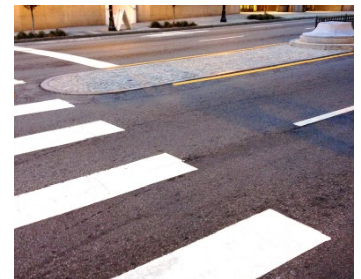
A flush median is recommended where trucks might otherwise run over a raised refuge
