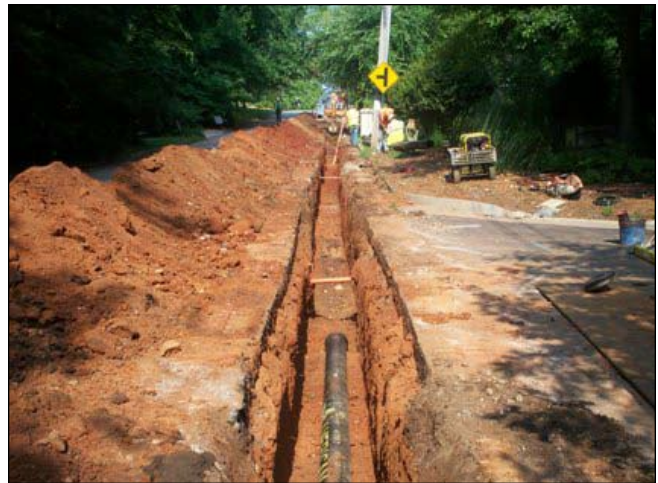
Aging sewer and water lines within the neighborhood are scheduled for evaluation and replacement where necessary
