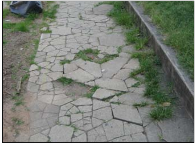
Broken sidewalks are a problem on some neighborhood streets, as shown in orange below
