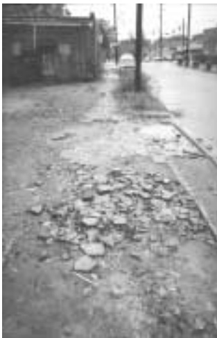
Figure 2: 3 Broken sidewalks are a public safety concern, discourage walking, and contribute to visual blight.
