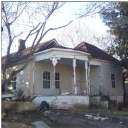
"Deteriorated" building condition
