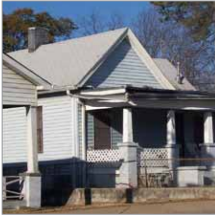
"Substandard" building condition
