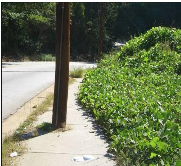
Utility poles and overgrown vines can reduce the usable width of a sidewalk.
