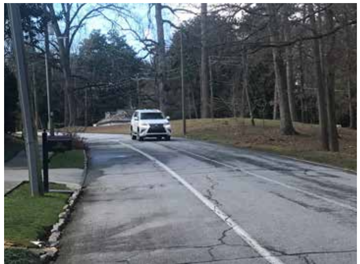
Vehicles speeding eastbound on Peachtree Battle Avenue often use unprotected bike lane.
