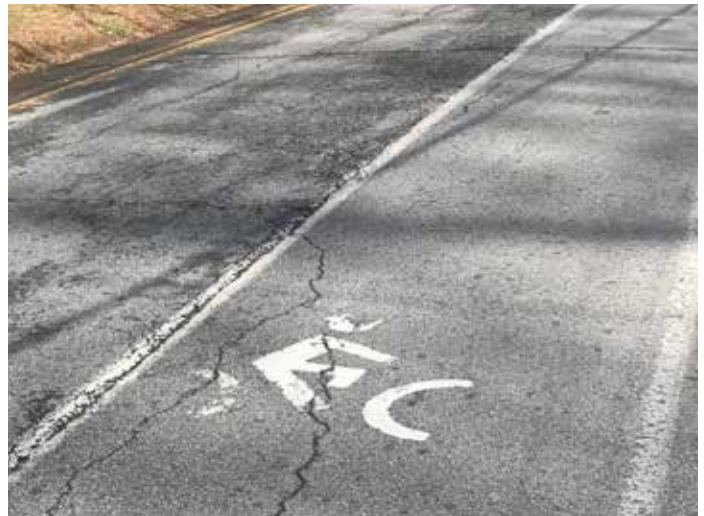
Bike lanes on Peachtree Battle Avenue are faded and lack markings in many locations.
