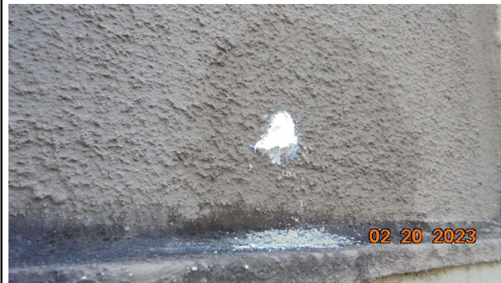
General Photo of sample location after patch
