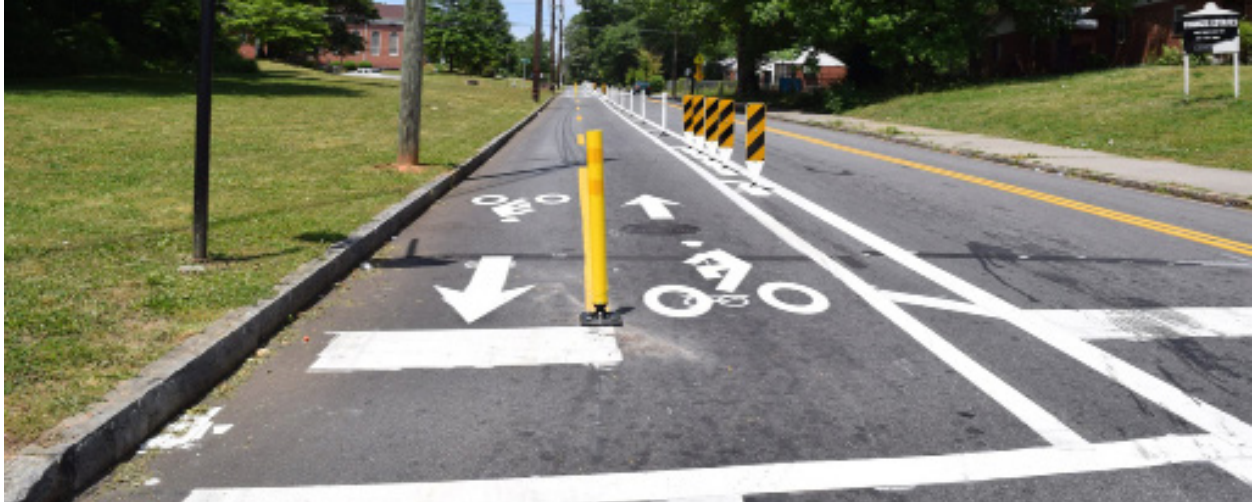
The Westview Drive two way protected bicycle facility was installed during a typical resurfacing project.
